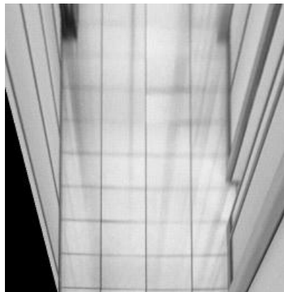
Warped: floor tile square
